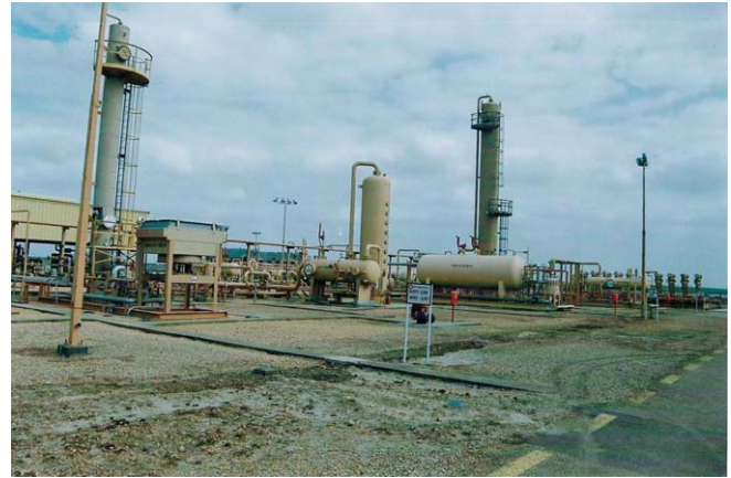
Gas processing plant in Nara Desert, Pakistan.
