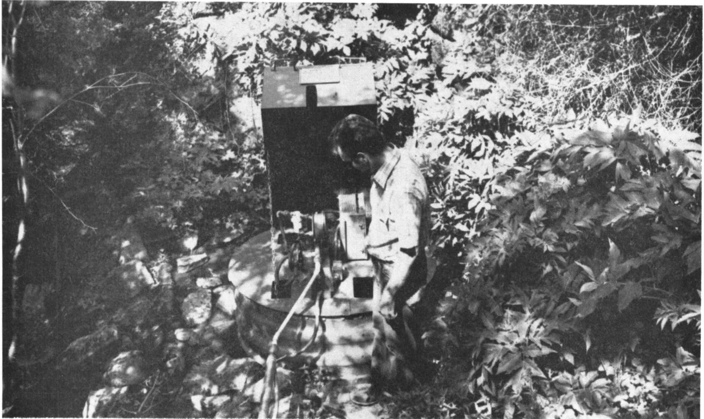
Dave Stevens observing the spring box, transformer and pump at Gibbler Spring.
